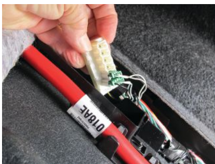
This is the connector that I tried to hook up to while working by flashlight. The proper connector is green.
